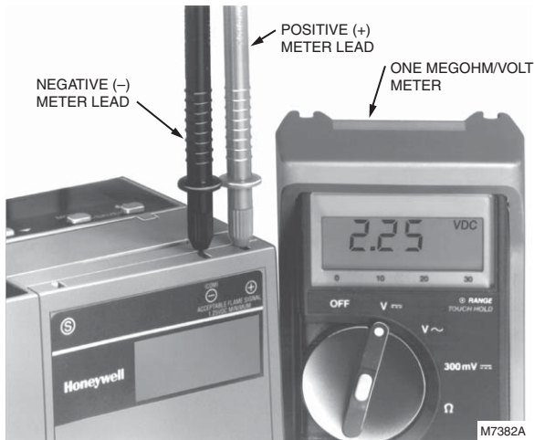
Fig. 11. Measuring flame signal voltage of 7800 SERIES controls.
